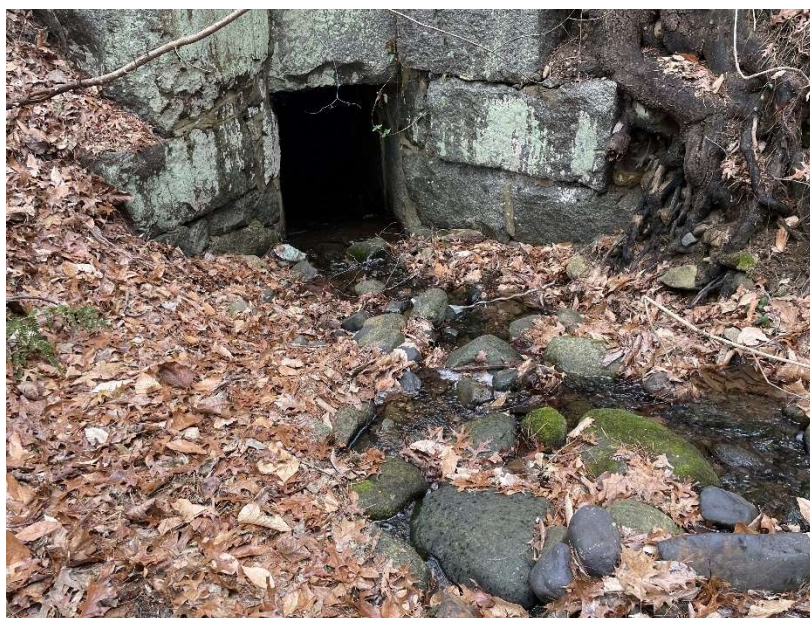
There are several existing stone block culverts along the corridor which facilitate storm water flow.
